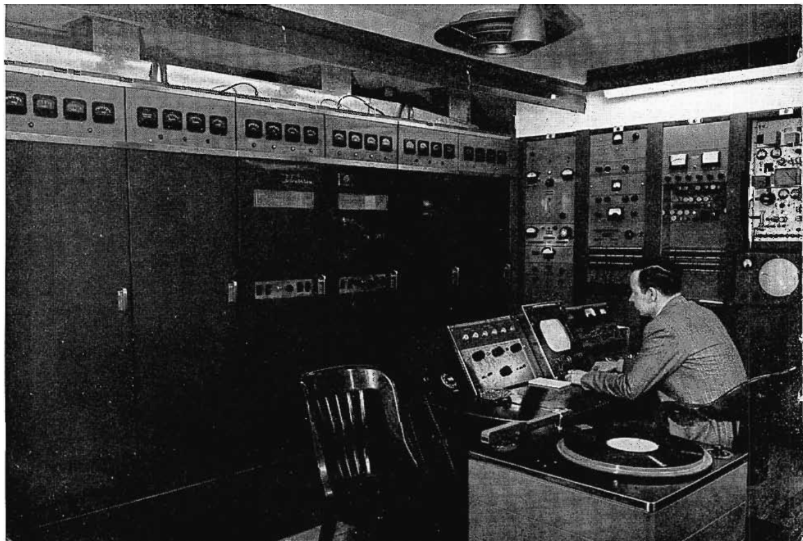
FIG. 3. View inside the transmitter room showing the RCA UHF transmitter, control console and monitoring racks. Transmitting equipment requires little floor space and rivals commercial TV installations in appearance. Seated at the console is Victor Bary, Senior Station Engineer, NBC.
